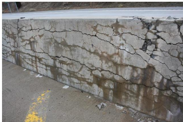
Figure 2. ASR damage in highway barrier (Deschenes Jr., 2017)
