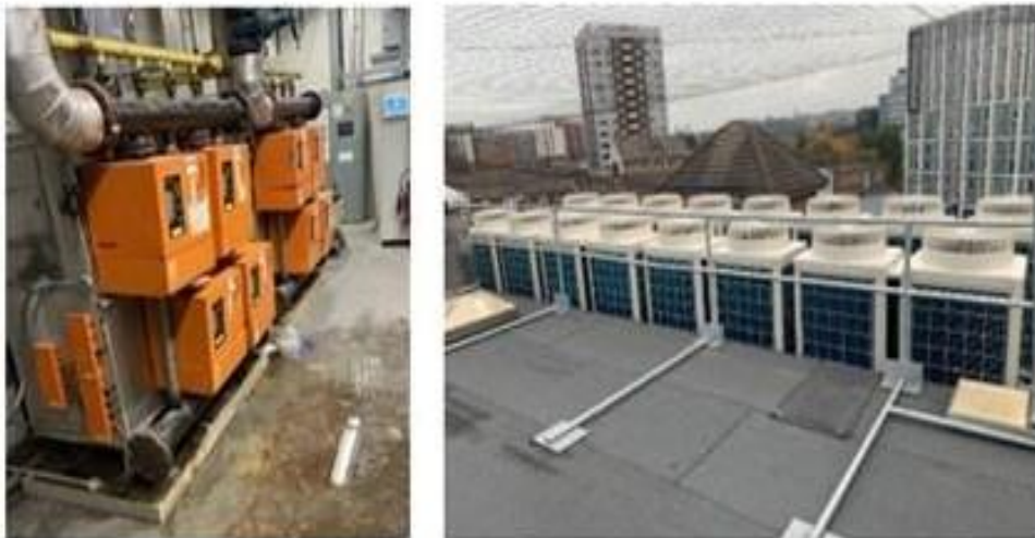
Figure 3. Space requirements for boilers and air source heat pumps Henry Cotton
