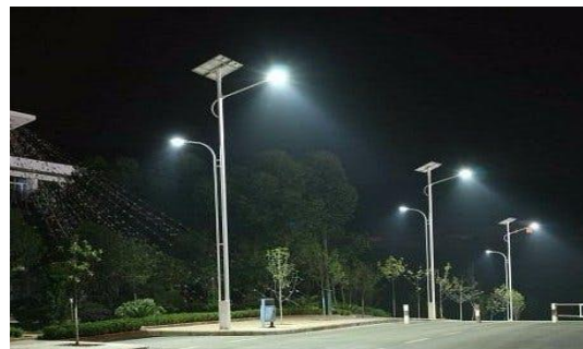
Fig. 1 Smart Street Light System
